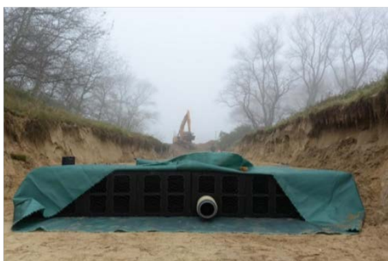
Figure 4 (a) Construction of 'subterranean infiltration' in water catchment of St-André (Koksijde). © IWVA
