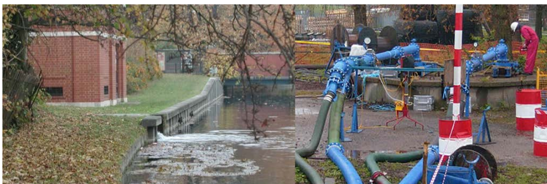
Figure 3. Test pumping an old, large diameter well in 2000 at 20,000 m 3 /d, and a modern NLARS borehole building with discharge into the New River. © Thames Water Utilities Ltd
