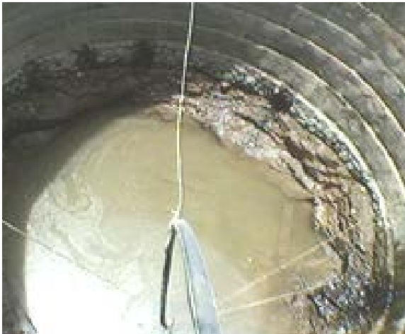
Low water level of well near check dam in summer season
