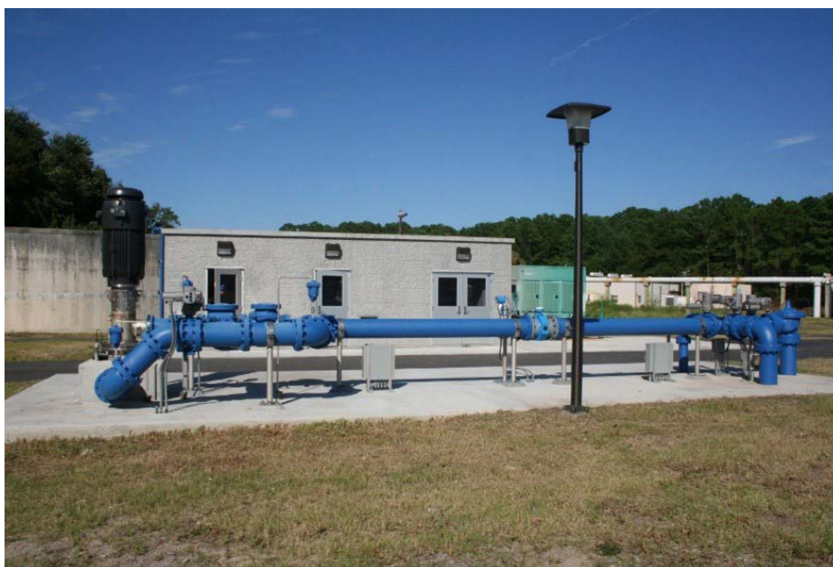
Figure 1. Well ASR-1 at Royal James, with pump, motor, wellhead piping, equipment shelter for electrical and SCADA controls, disinfection and emergency engine. © David Pyne
