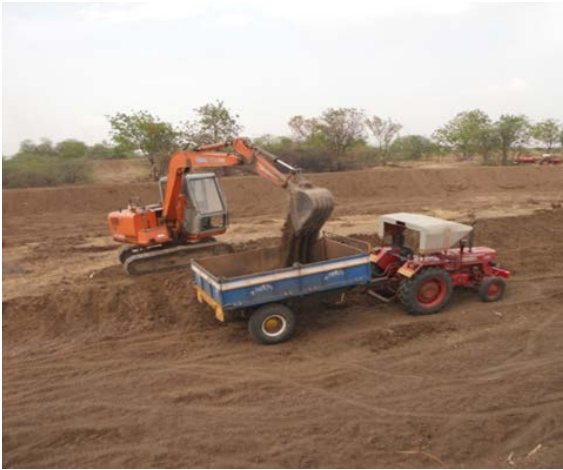
Removal of tank silt from check dam in Jalgaon K.P. NICRA village.
