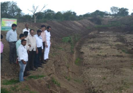
After removal of silt from check dam in Jalgaon K.P. NICRA village.
