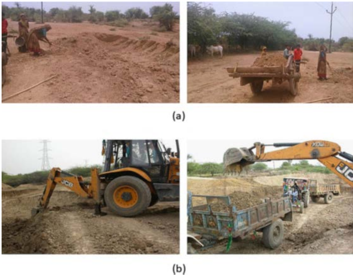
Figure 3. Desilting methods used for check dams before the 2015 and 2016 monsoons: (a) manual desilting of Badgaon check dam before 2015 monsoon, (b) mechanical desilting of Hinta check dam 2016. © Yogita Dashora
